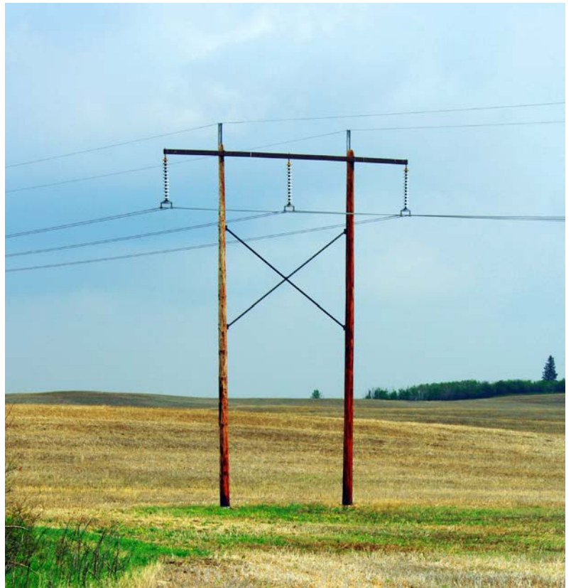
Typical H-frame structure (final design may vary) . Most of the line will be built with two H-frame structures side by side. Non-typical structures including mono poles and lattice towers may be used.
