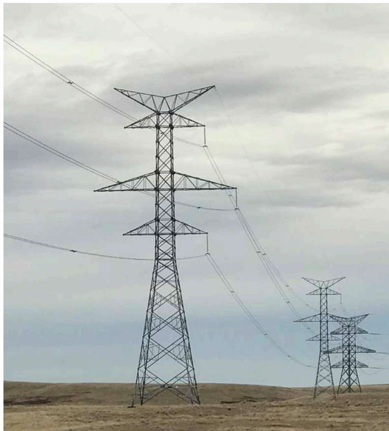
Typical Double Circuit Steel Lattice Tower (final design may vary). This project will have a single-circuit steel lattice tower.
