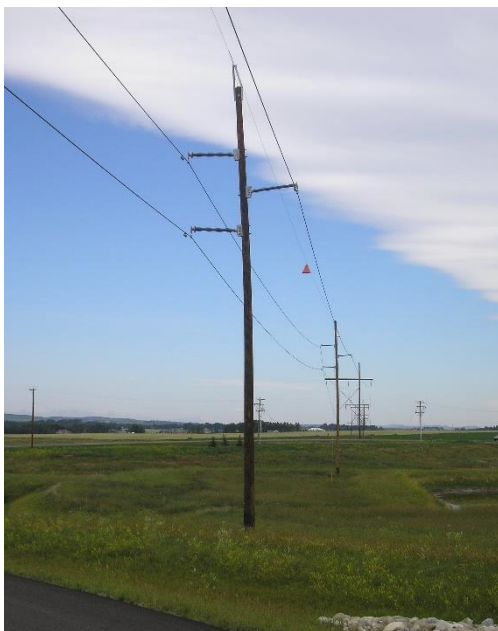
Above: A typical 138 kV structure. The rebuilt structures will look similar.
