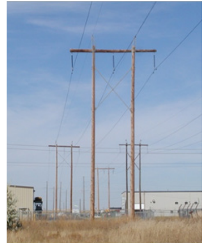
The existing 892L transmission line.
