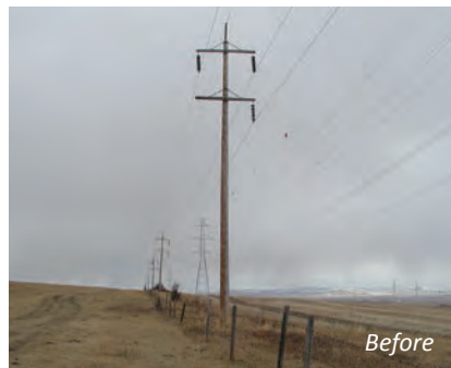
After Photo of 138 kV double circuit mono-pole structure similar to structures being proposed
