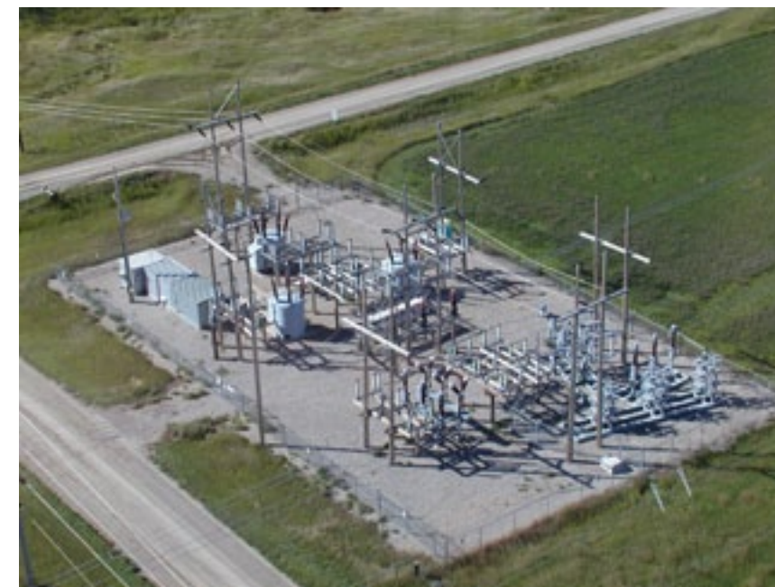
Existing Blackie Substation
