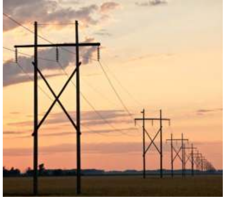
Stock photo for illustrative purposes - typical transmission line
